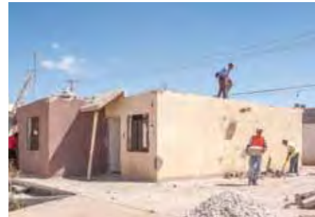
Retiro de blocks al área de clasificado del material desmantelado. Removing the blocks to the area of classification of the dismantled materials.
