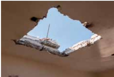
Vano en losa de la azotea. Opening in the floor of the flat roof.
