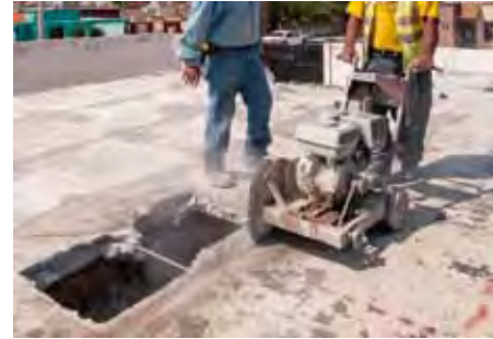
Hueco en losa de azotea con máquina cortadora. Opening in the floor of the flat roof with cutting machine.
