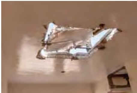
Proceso de abertura de losa en la azotea. Process of making an opening in floor of the flat roof.
